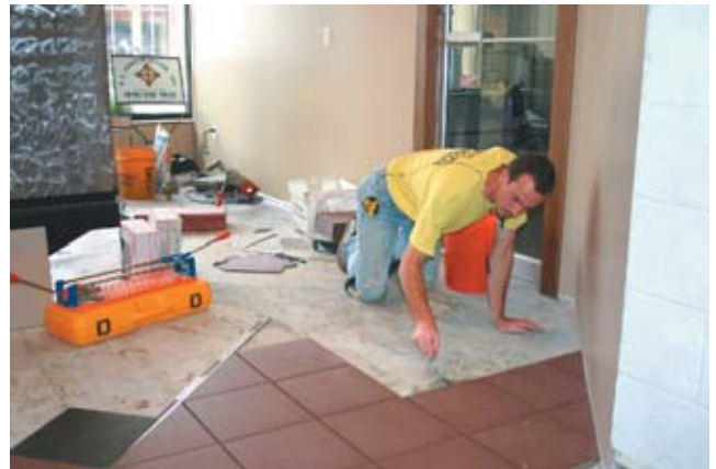
FLOORED -- Independent contractor Marc Briggs prepares to add another row of tile to the floor of the INA/INF building front entry. The remodeling project is nearing completion.
